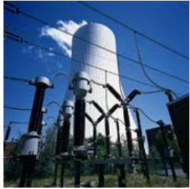
Power Generation and District Heating
